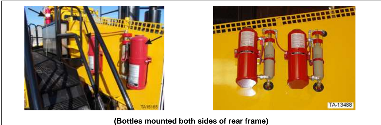
Figure 42. Fire suppression system bottles - AFEX system shown
