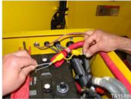
Fire suppression in-line fuse located in loader battery box.
